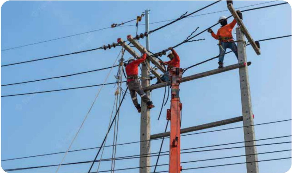
Overhead Electric Cable Line
