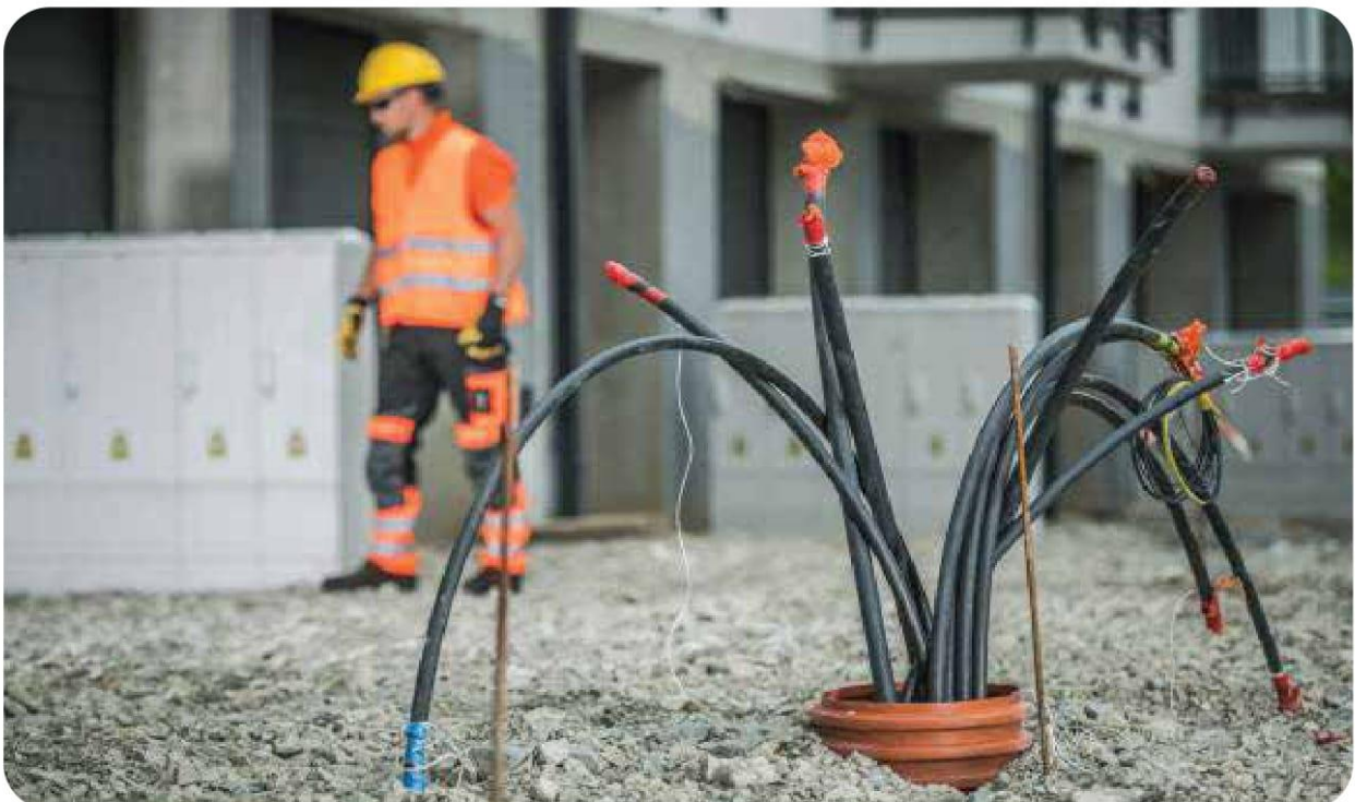
Underground Electric Cable Line
